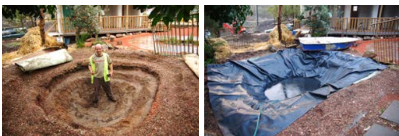
Shaping the pond, laying pond liner and filling the pond with on site rain water.
