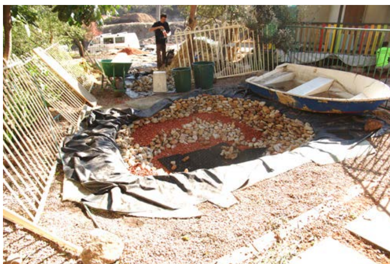
Rocks and crushed tiles stacked to emulate a natural pond, however no soil or mud used Black Atlantis drain cell in bottom of pond to protect liner while we worked was found on site note the change in the toilet hand rail
