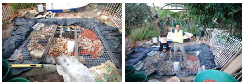
Installing and testing child safety cage for OH&S, hardwood beams, cage (school fence) and construction safety fence (old pool fence) were sourced from the Buy Back Centre, recycled Timber Yard and ANL all within 100m of the site
